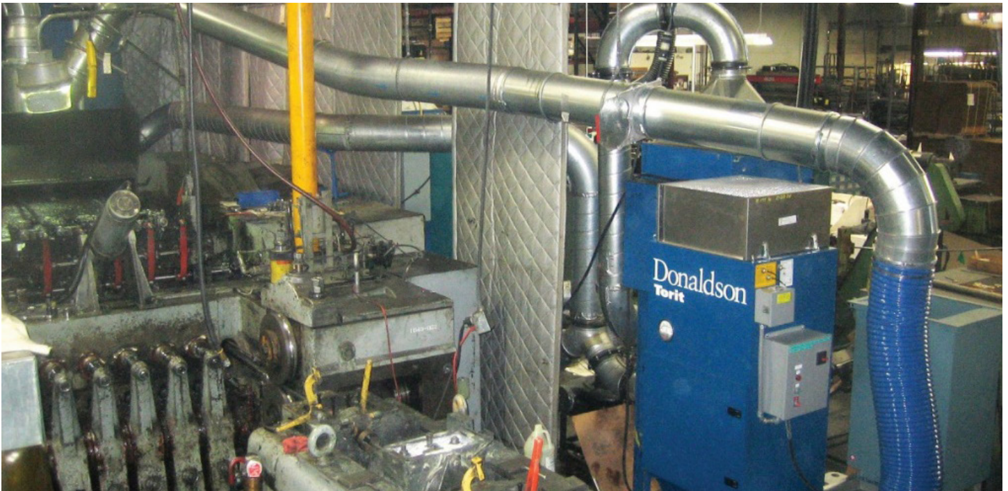
Figure 1: Donaldson Torit WSO Mist Collector capturing smoke.
