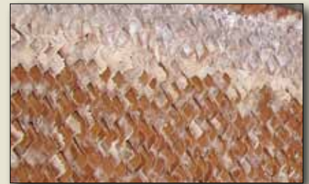
Scaling or "white frost" on evap media surface.
