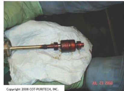
Fouled Oil-Level Sensor
