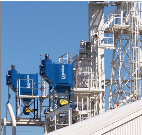
Two Donaldson Torit Downflo Oval (DFO) dust collectors have a small footprint and yet are sized for the high airflow needed for eight concrete color holding tanks.
