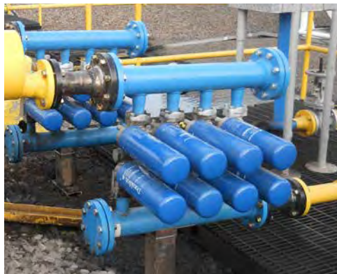
Single-pass Bulk Fuel Filtration System
